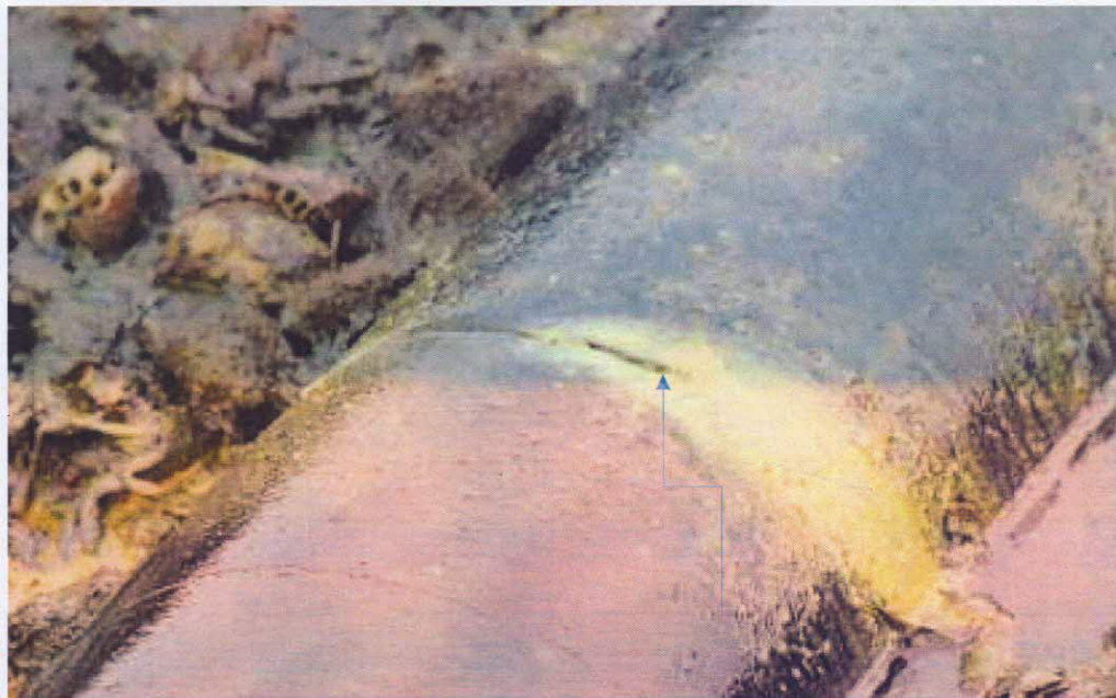
HACKSAW CUT AT 12 O'CLOCK POSITION ON THE FLOWLINE.
